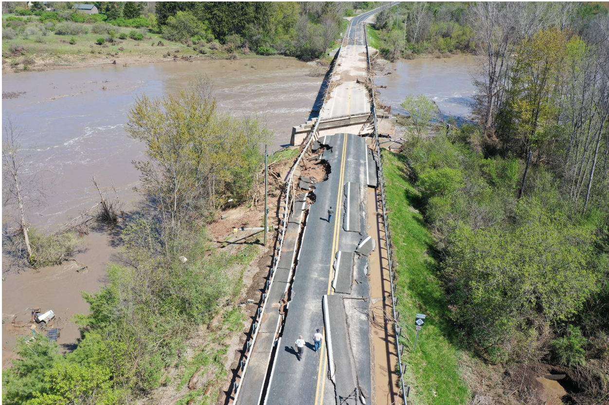
Figure 4. Roadway Flooding in Midland County, Michigan
